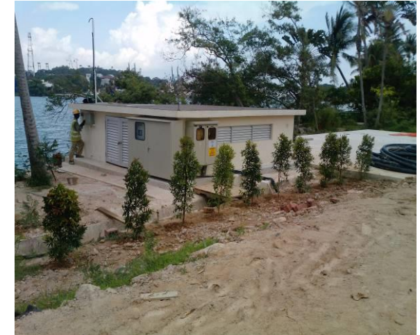
IRRIGATION PUMP STATION AND STORAGE TANK AT SENTOSA GATEWAY
